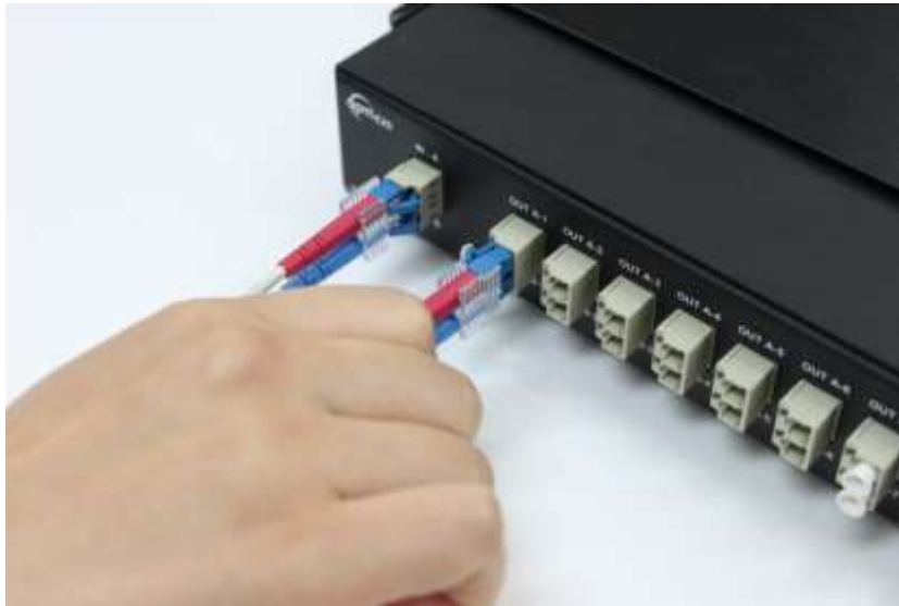
Fig. 8: LC patch cord into output receptacle
